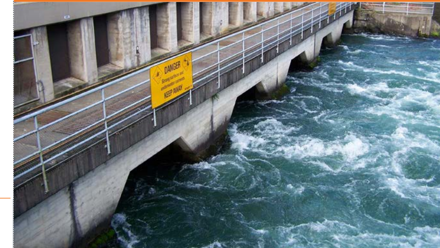
JOHN HART DAM & GENERATING STATION, Campbell River, BC BTY Group is providing Cost Consulting services for this P3 project.
